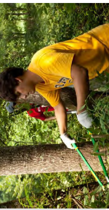
Planned greenway corridors are oftentimes overgrown with weeds, trees and other foliage and need to be cleared not only for trail establishment but to promote safety and visibility along a route.
